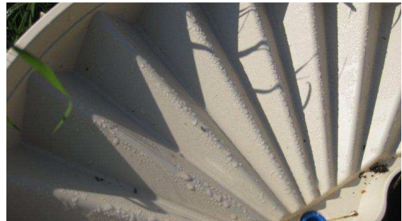
Condensation effect on top of the Waterboxx
